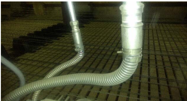
BROKEN CABLE CONNECTORS
