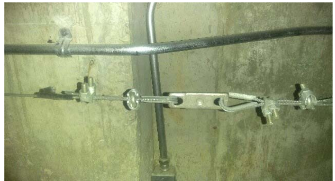
FIRE CURTAIN: IMPROPER TERMINATIONS
