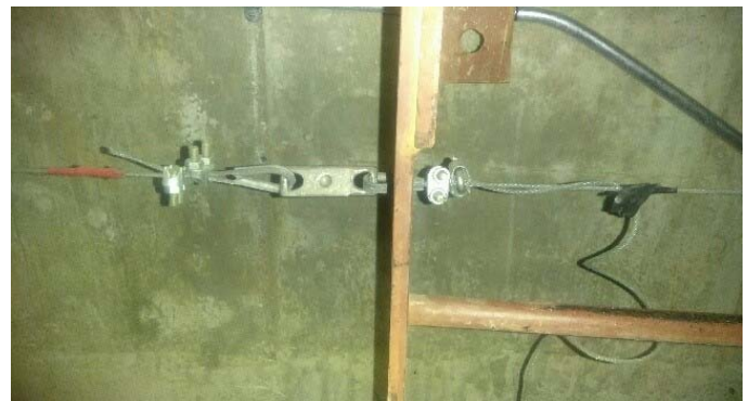
FIRE CURTAIN: IMPROPER TERMINATIONS
