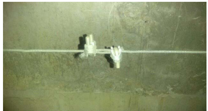
FIRE CURTAIN: IMPROPER TERMINATIONS
