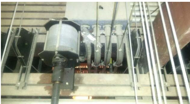
BROKEN CABLE PROTECTOR
