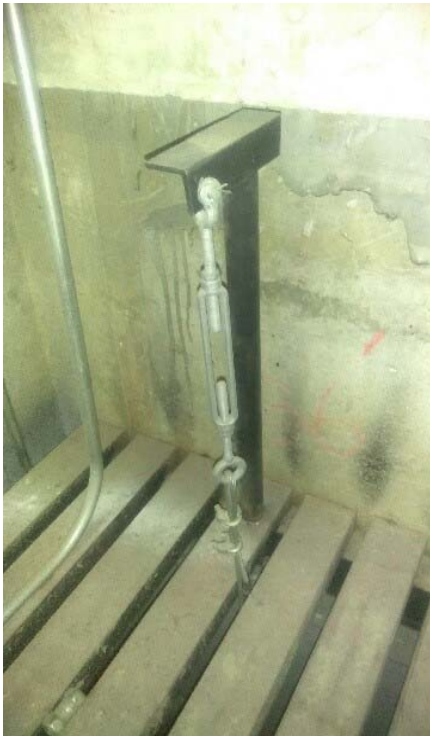
TURNBUCKLES FOR FIRE CURTAIN NOT MOUSED
