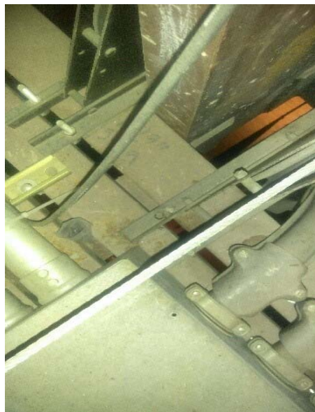
MISSING/LOOSE J-BOLTS & U-BRACKETS
