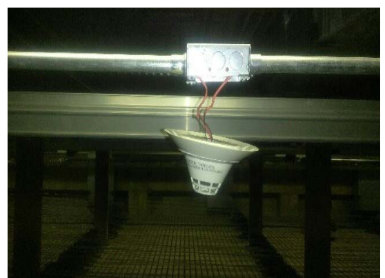
BROKEN FIRE SENSORS
