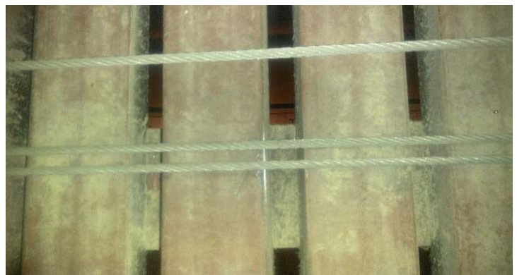
CABLES RUBBING GRID
